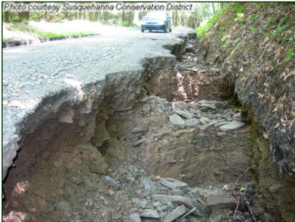
A badly eroded ditch on its way to a nearby stream
