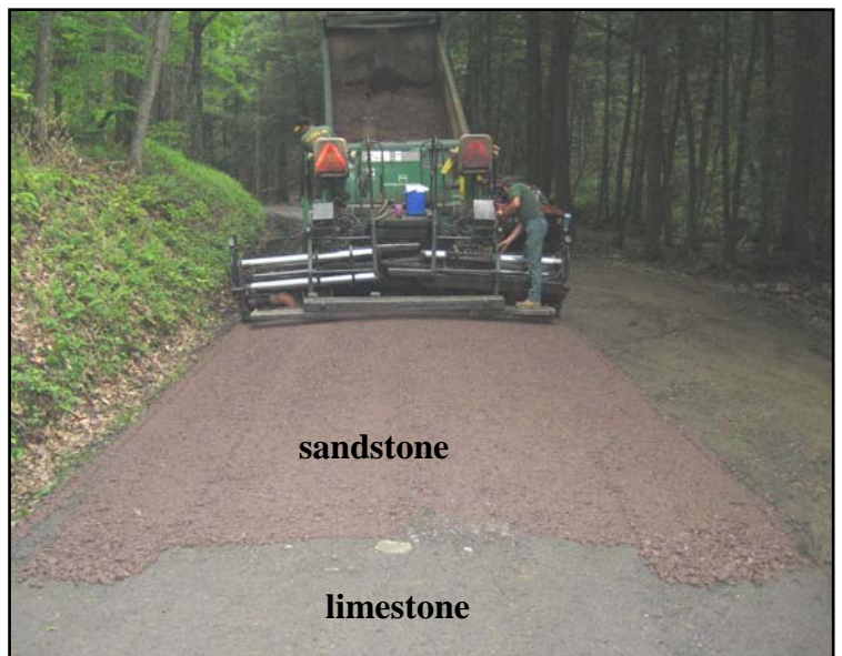
Figure 2.4: A motor-paver places DSA on Lebo Road in Potter County. Lighter colored limestone DSA is in foreground, while reddish sandstone DSA is being placed by the paver.
