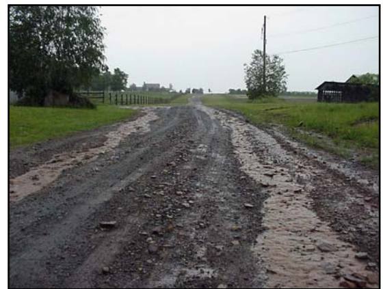
Figure 4.2: Grade breaks are designed to prevent erosive flows of water on the road surface like the one pictured here.
