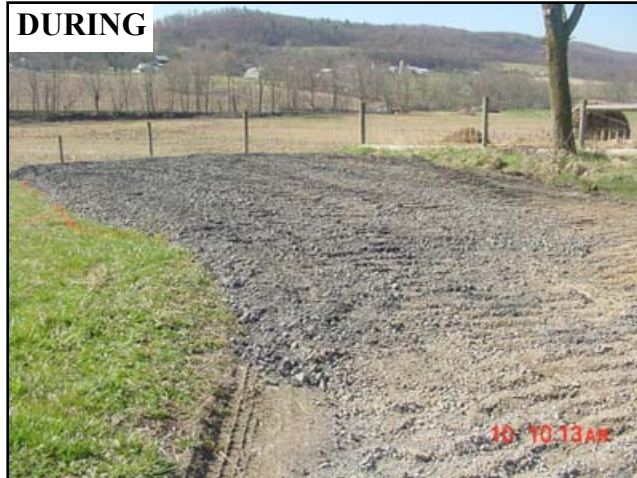
Figure 4.16: A broad-based dip is being constructed just before a steep part of the lane. The dip will divert water into the field instead of allowing it to flow down the road.
