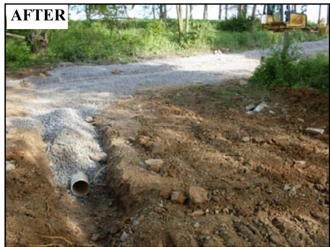
Figure 4.10: The outlet of the stone underdrain is shown here just after installation. The underdrain collects clean subsurface water before it enters the road area.
