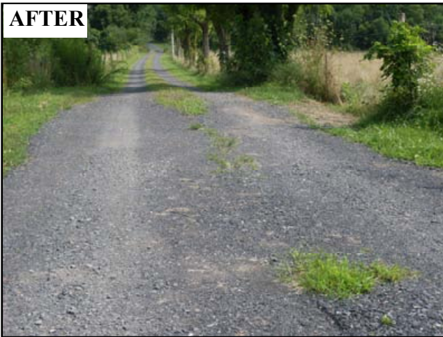
Figure 4.20: The gradebreak pictured here sheds water from the road surface, preventing it from flowing to the bridge and stream in the background.
