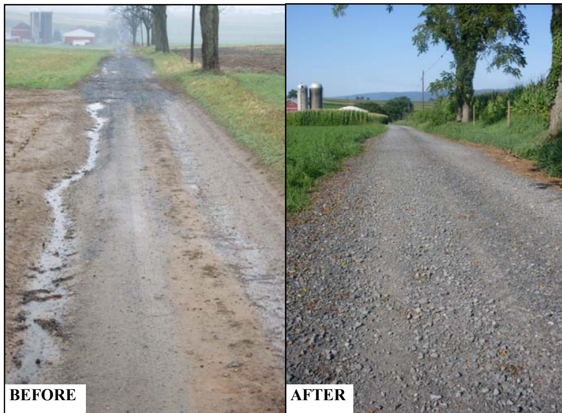
Figure 1&2: BEFORE the project, the entrenched farm lane collected field runoff and transported it down the road surface. Many practices were implemented to elevate the road, encourage infiltration, and insure that runoff could no longer use the road as a flow corridor.
