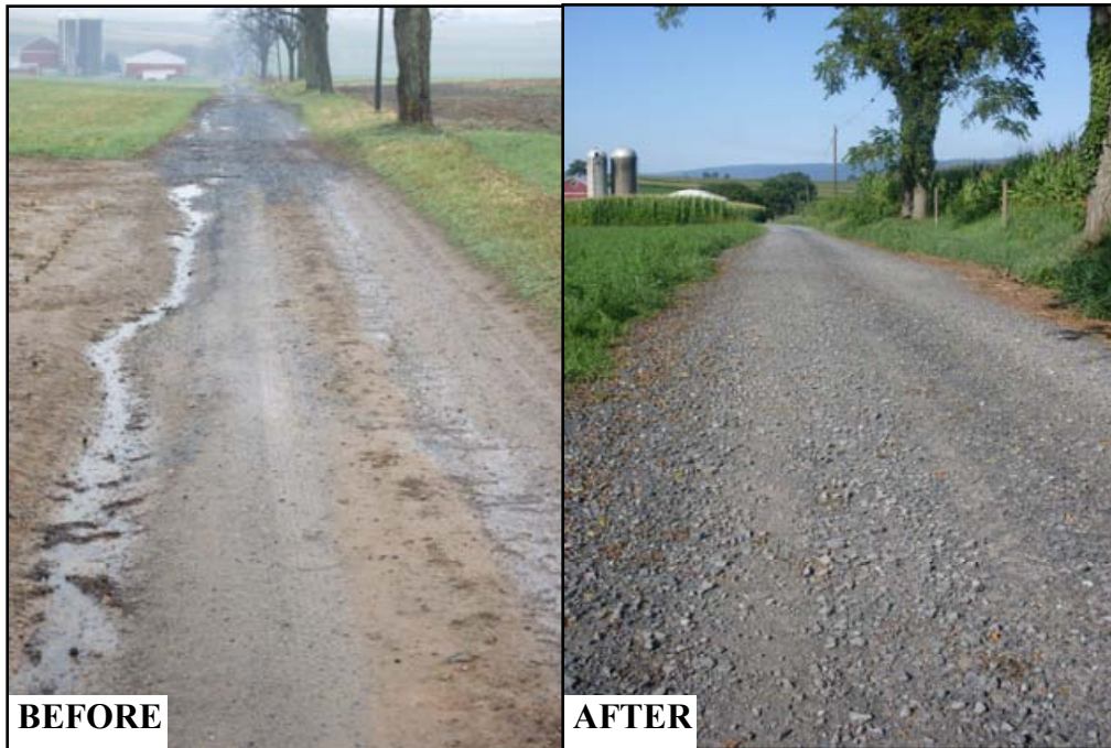
Figure 4.6: BEFORE the project, the entrenched farm lane collected field runoff and transported it down the road surface. Many practices were implemented to elevate the road, encourage infiltration, and insure that runoff could no longer use the road as a flow corridor.
