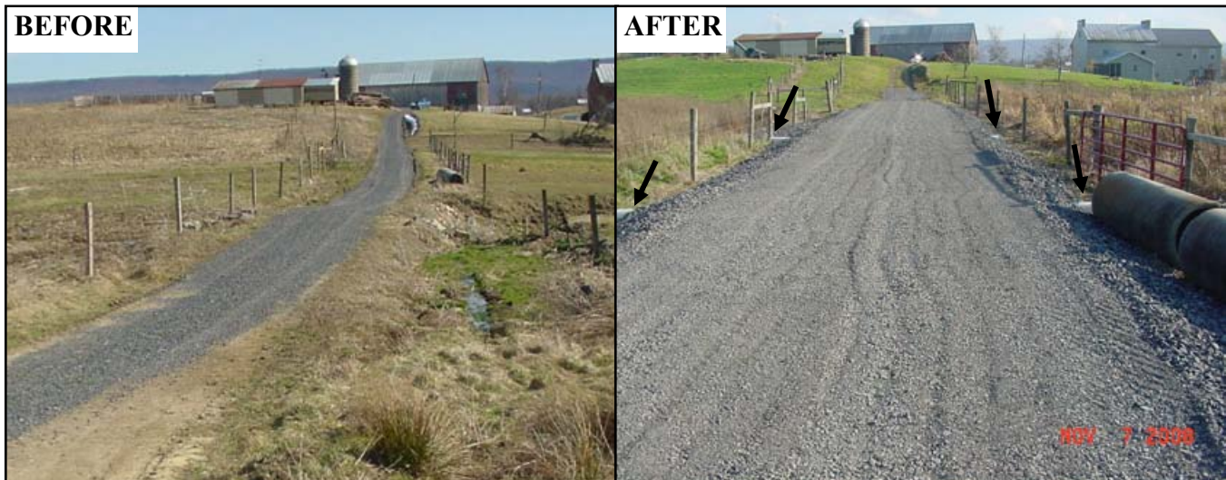
Figure 1: This is the wetland stream crossing on the Goss Farm. Notice that BEFORE, water is dammed up against the right side of the road and funneled through a single pipe. The AFTER picture shows the 120 foot French mattress. White relief pipes are visible and highlighted with black arrows. Notice also that the road's "lowpoint" has been moved away from the stream so runoff is forced to leave the road before nearing the channel. The Broad based dip at this location forces the water to the down slope side of the road.
