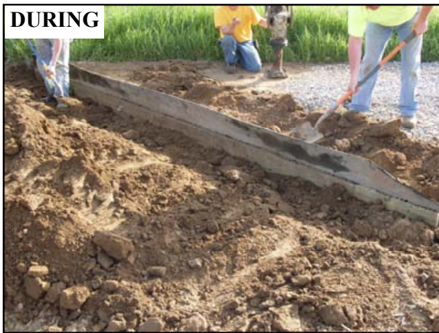
Figure 4.9: A conveyor belt diversion is being installed across the road that will allow traffic to pass while diverting water off the road surface.
