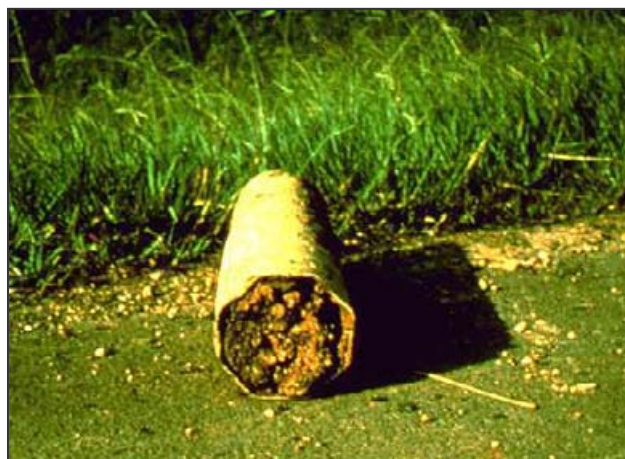
Fabric and outlet protection are important to prevent clogged pipes such as this.
