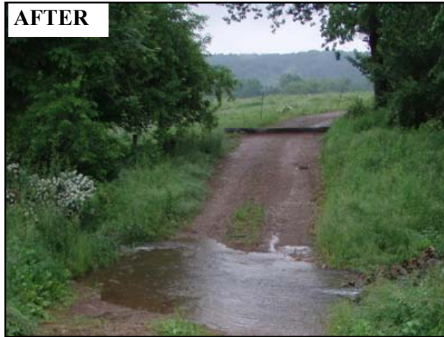
Figure 4.13: A conveyor belt diversion, installed before the ford crossing, insures runoff is diverted before it can reach the stream.
