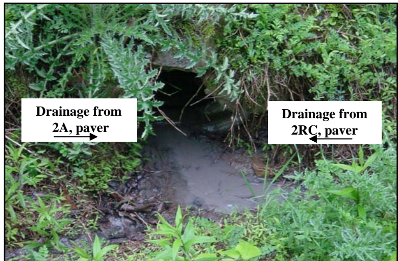
Figure 17. This culvert is located at the boundary of two aggregate placements. Clear runoff on the left of the image is runoff from “Section 5: 2A, Paver.” The sediment-laden water on the right of the image is runoff from the clay containing aggregate on “Section 4: 2RC, Paver.”
