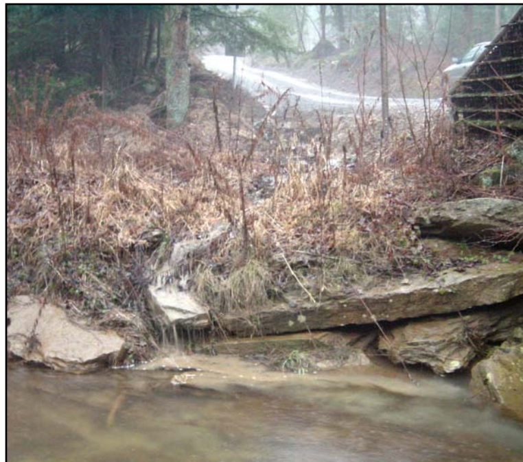
Figure 1. Ditches from the unpaved road in the background dump sediment into a High Quality stream at a bridge crossing near Clarion, PA.
