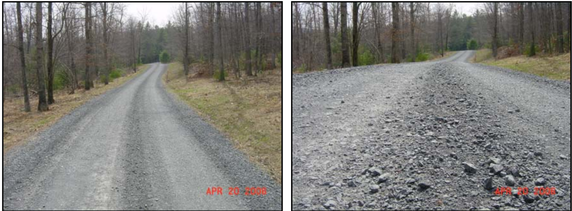
Figure 15. Section 5, 2A paver-placed, shown in April of 2006. More pictures located in Appendix C.
