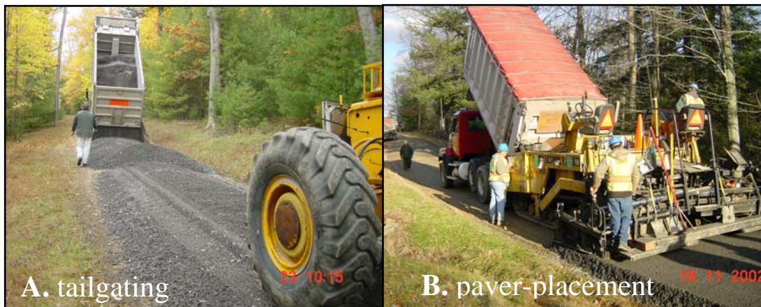
Figure 2. Photo “A” on the left illustrates the process of tailgating aggregate. A windrow of aggregate has just been dumped out of the truck. A motor-grader waits to spread the material and shape the road. Photo “B” on the right illustrates the placement of aggregate through a paver. The truck is dumping aggregate directly into the paver which uses an auger to minimize segregation as it places material on the road.
