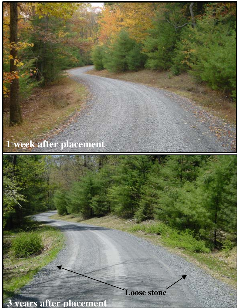
Figure 19. “Section 2: 2A, Tailgated” illustrates the outward migration of larger size aggregate. Larger stones are mobilized and windrowed on the centerline and shoulders of the roadway.
