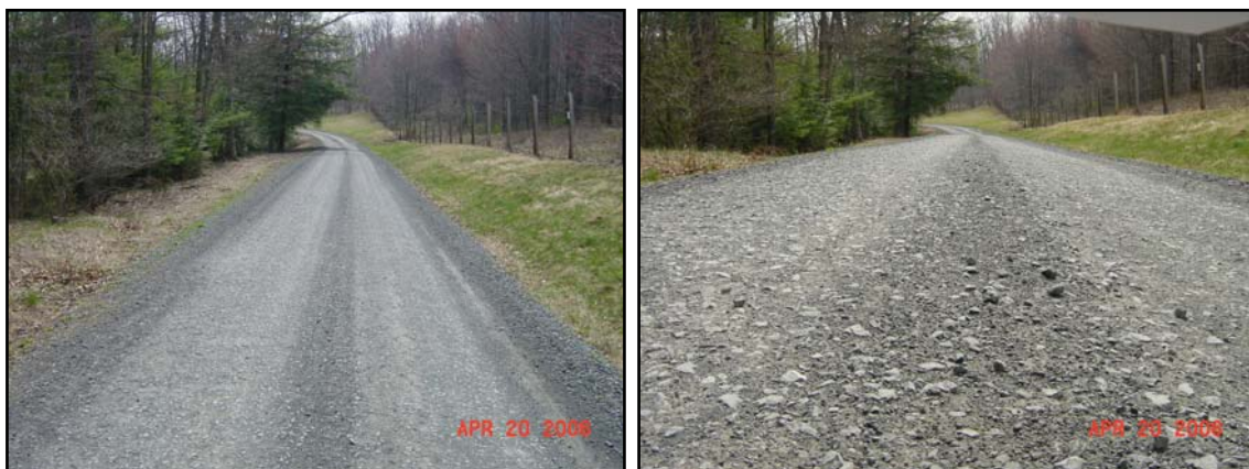
Figure 16. Section 6, DSA paver-placed, shown in April of 2006. More pictures located in Appendix C.
