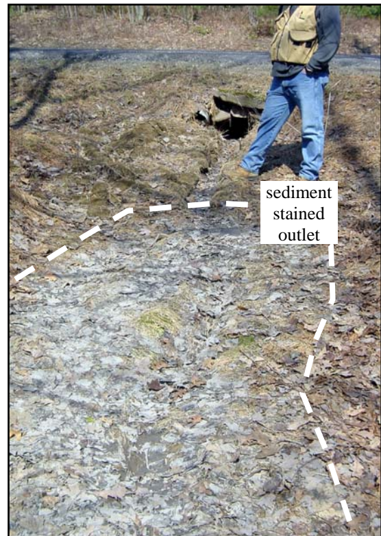
Figure 18. This culvert outlet located on “Section 4: 2RC, Paver” is visibly stained with sediment from runoff. Other aggregate sections had minimal visible sediment or outlet staining.
