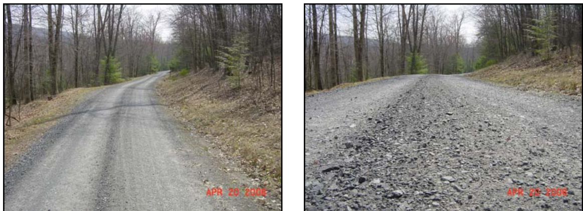
Figure 13. Section 3, DSA Tailgated, shown in April of 2006. More pictures located in Appendix C.
