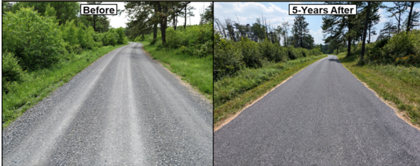
Figure 1. Conversion of a high traffic gravel road to a chip sealed road using AASHTO #67 aggregate base followed by a double coat of AASHTO #8 aggregate.
