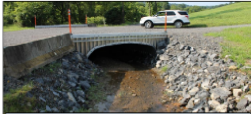
North Ridge Road, Iermanagh Township. DGR Project replaced undersized, double pipes with a 15" x 53" aluminum plate arch box culvert. Total project value: $121,000. DGR Grant: $100,000, Township Funds: $21,000.
