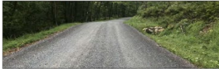
Cold Springs Road, Dickinson Township: Driving Surface Aggregate (placement 2019) and shallow cross pipe (installed 2017).
