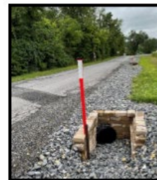
Cross pipes are commonly used in DGLVR projects to direct water away from the road and nearby streams.
