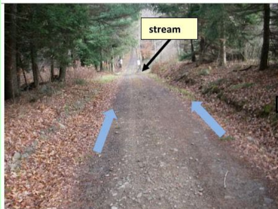
BEFORE: Entrenched road draining to stream.
