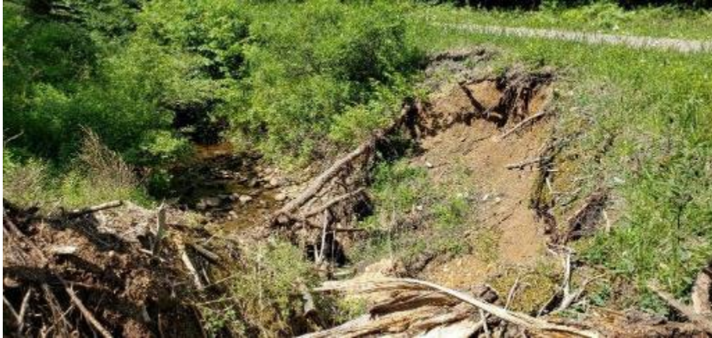
Slip Encroaching on Road
