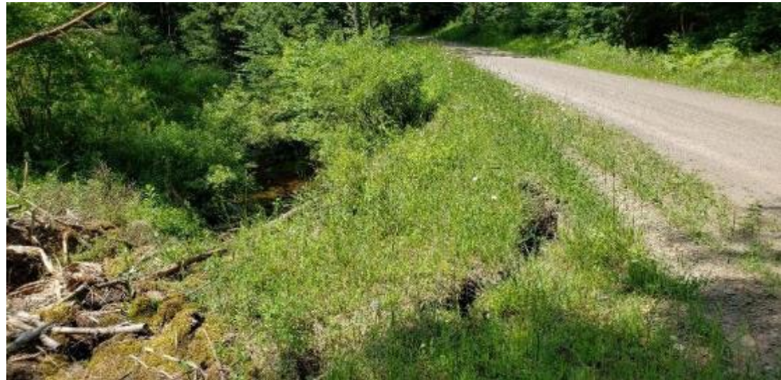
Road Bank / Stream Bank Failing
