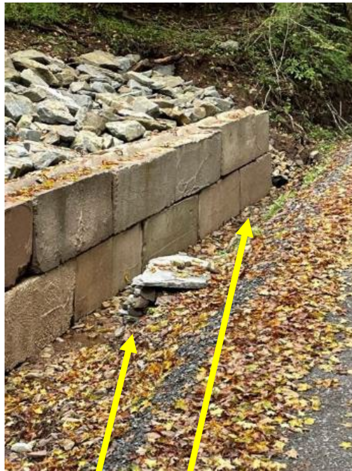
Footer drain and pipe remove water
