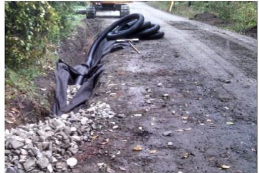
Photo 1: The ditch was always wet from roadside springs. This underdrain will collect spring flow to keep the roadbed and ditch dry.
