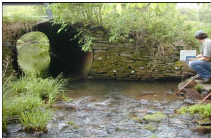
Photo 2. A stream passes through an old metal culvert.
