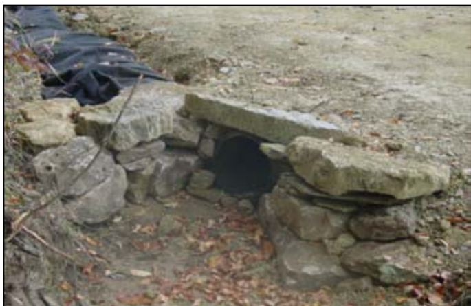
Photo 1. A plastic crosspipe is used to convey ditch flow under the roadway
