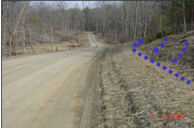
Photo 1 - A bank bench on Red Rose Rd., Huntingdon County, just after construction. This bench is one width of the backhoe bucket and was constructed from the road way.
