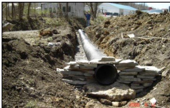
Photo 1. A plastic crosspipe is shown during installation. Notice the pipe bedding material, endwall, and stone at outlet.
