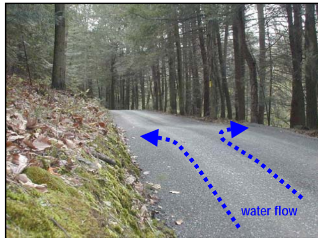
GRADE BREAK – Interruption in slope redirects flow and causes water to leave road area.
