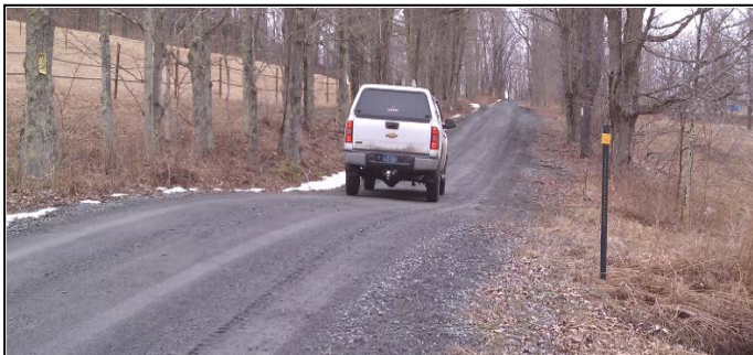
Grade Break - A small increase in road elevation on a downhill slope, which forces surface flow off the road.
