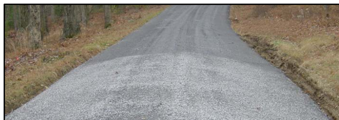
Center Crown – High point on road centerline with 4% to 6% slope to road edge ( \frac{1}{2} " to \frac{3}{4} " fall per 1' lane width)
