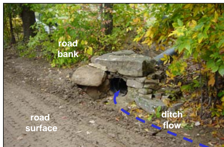
Photo 2. This is the inlet of the same “through-the-bank” pipe shown in Photo 1. The pipe has just been placed and is about to be covered.
